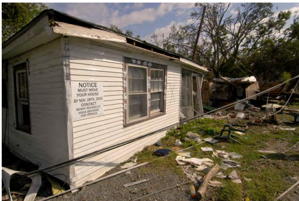
Sign posted by Parish officials warns homeowners of pending demolition if their house is not moved. Marvin Nauman / FEMA
