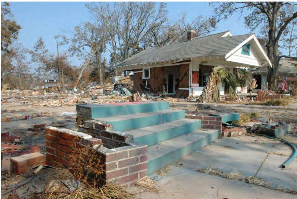
While Hurricane Katrina pushed many houses off their foundations, it usually was impossible to prove whether the damage was due to wind or flooding. The distinction is critical when claims are filed with insurance companies. Mark Wolfe / FEMA
